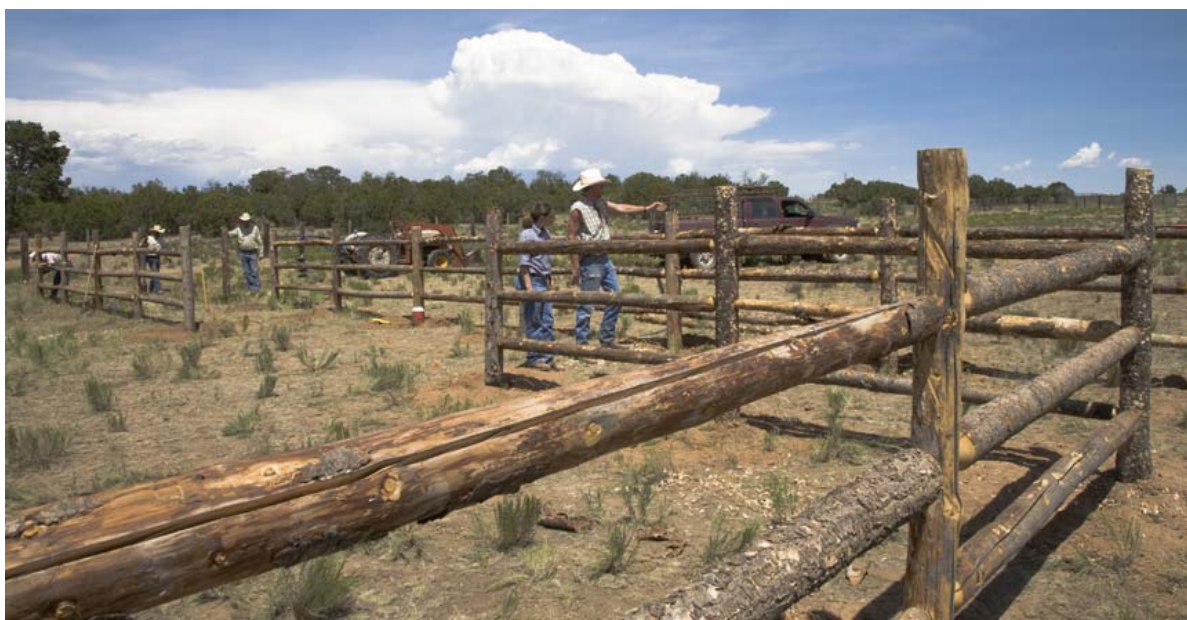
LMCC arena takes on a realistic feel as staff members construct pens for the upcoming sale on April 19, 2008.
